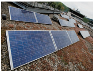
Solar panels installed at the Stuttgart Technology Center
