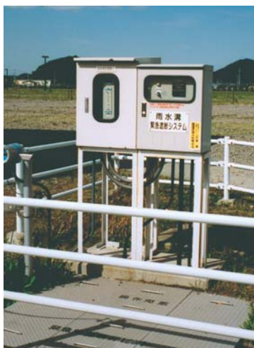
Rainwater Drain Emergency Shutoff System
